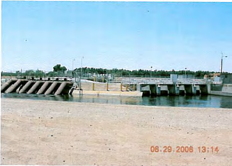
Permanent pumps in the Tule River Wasteway used to move water from the Tule River into the Friant-Kern Canal.
