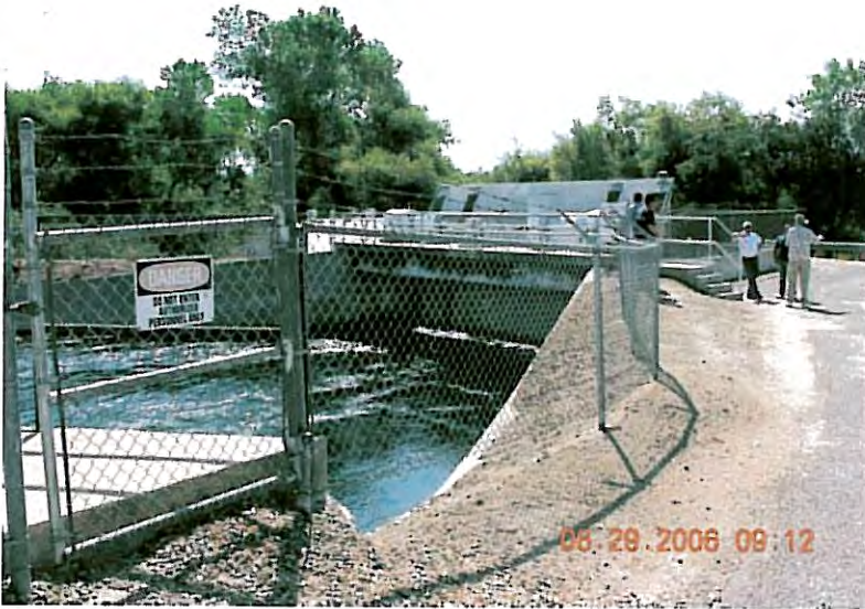
Friant-Kern Canal gate that moves water into Fresno Canal and the Kings River.
