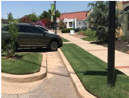
Figure 9. Large drainage channels increase the speed of water along Paseo and create trip hazards for pedestrians.
