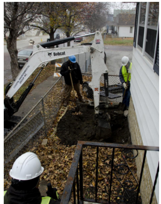
Excavation of lead contaminated soil at residence within the Omaha Lead Superfund Site
