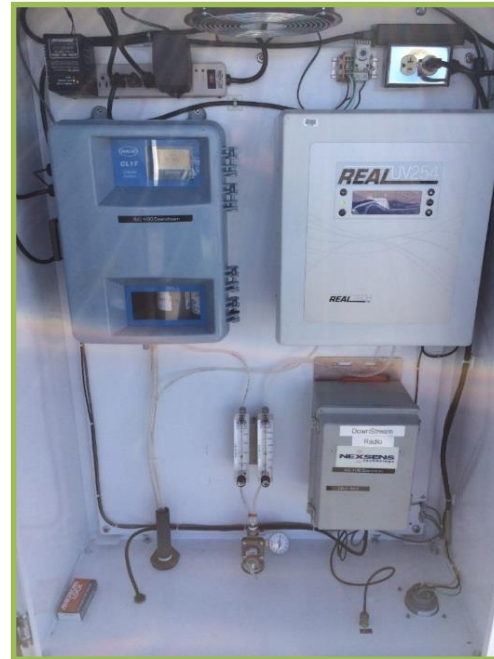
Chlorine and TOC Sensors with Cellular Modem
