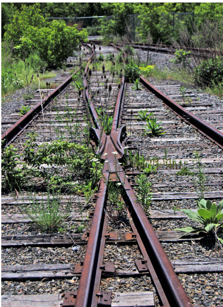
Site infrastructure that EPA left in place after cleanup included an on-site rail spur.
