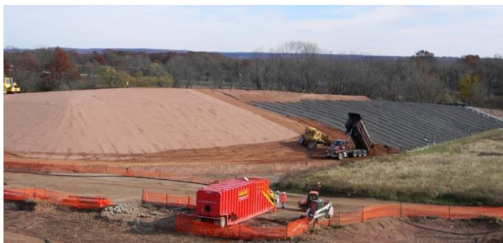
Above: Reuse of facility soil for grading significantly reduced the volume of imported fill material.
