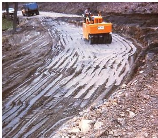
Highway embankment with fly ash structural fill. (U.S. Department of Transportation photo)
