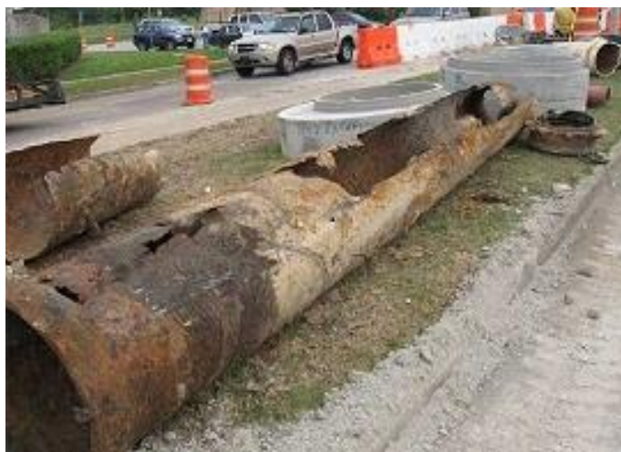
Repairs to a steel sanitary sewer force main in Houston. (Photo from city of Houston website)
