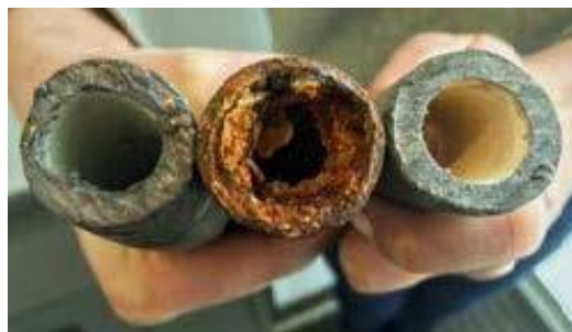
Lead service lines showing inner surface without any coating from corrosion control treatment (left), with coating (right), and fully corroded (middle). (EPA photo)
