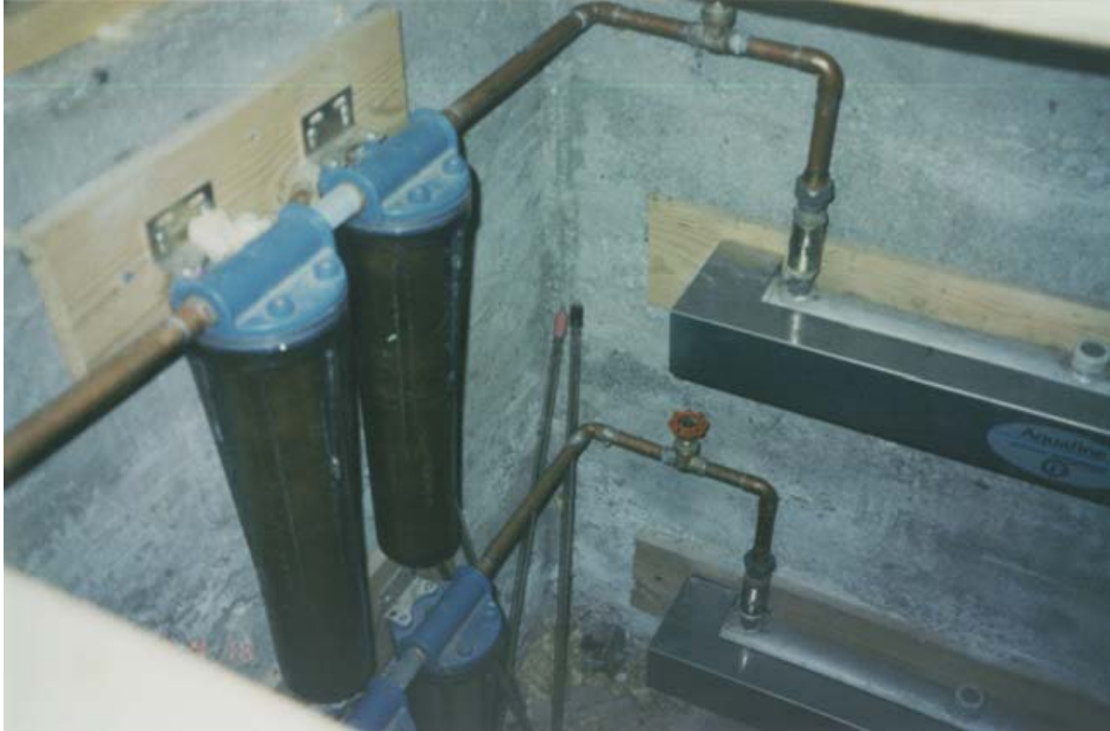
Figure 2-5. Cartridge Filters Installed at a Small PWS
