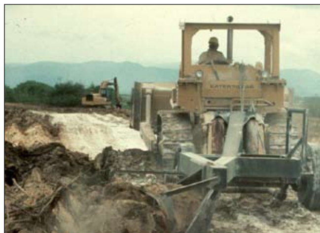
Deep plow tilling and incorporation of lime is an effective tailings remediation tool.
