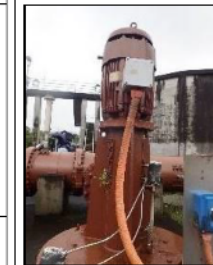
Hilo WWTP Biotower Pump No. 1 POF: 4
