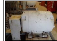
Hilo WWTP Headworks Blower No. 1 Motor POF: 2
