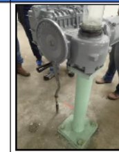
Pua Pump Station Discharge Valve No. 1 POF: 1
