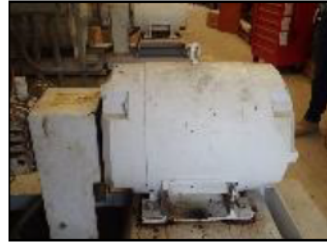
Hilo WWTP Biotower Pump No. 1
