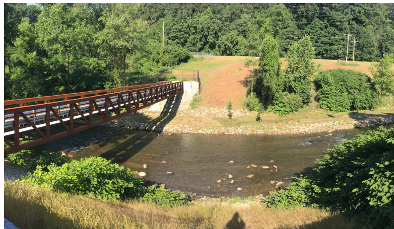
Uhler conveyance project and Little Cuyahoga River stream bank restoration. Photo courtesy of City of Akron.
