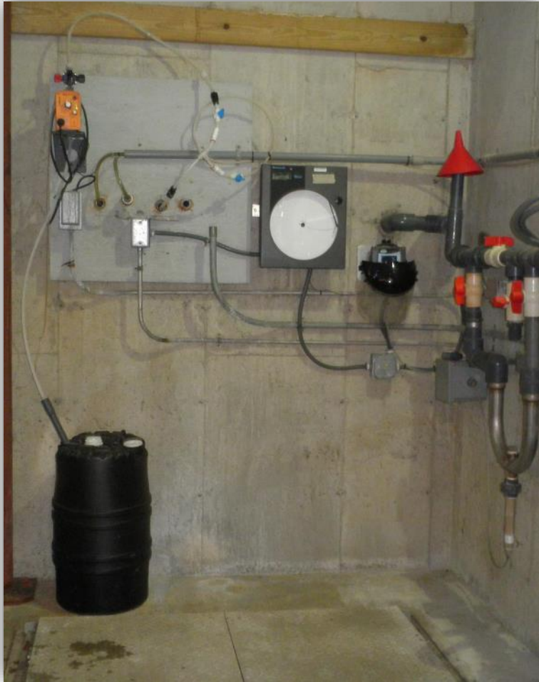
Alkalinity Control (Sodium Hydroxide)
