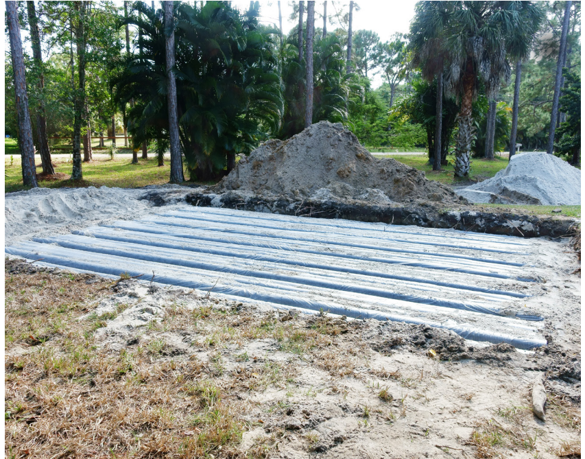
Image 2: Septic drainfield. (Photo courtesy of EPA)
