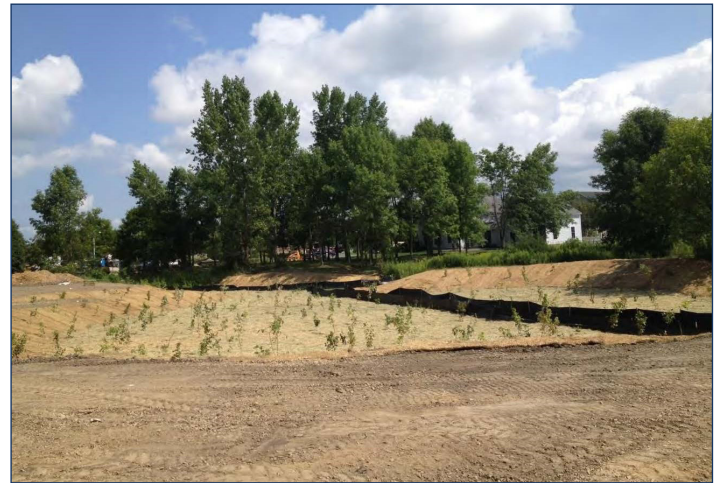
Image 36: Floodplain area directly after construction and planting of native tree and shrub species. (Photo courtesy of the final grantee report)
