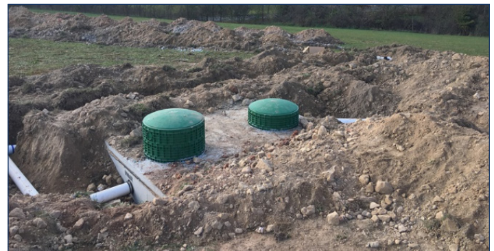
Image 37: Installation of an advanced treatment system. (Photo courtesy of Stone County Health Department)
