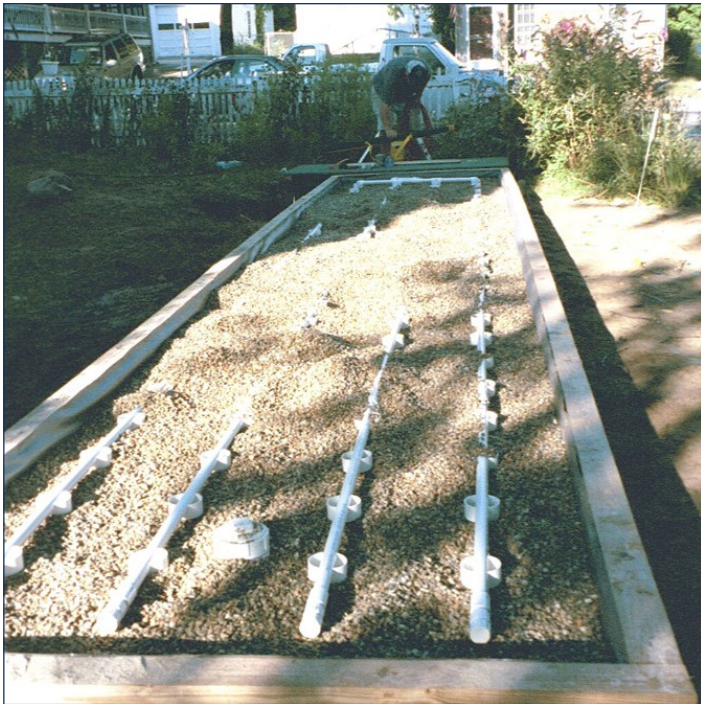
Image 15: Bottomless sand filter fits into a small space at a property on Main Street. (Photo courtesy of the final grantee report)
