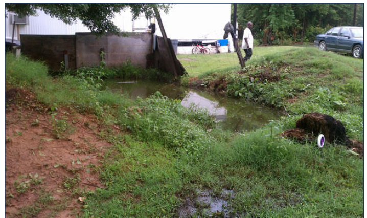
Image 25: A pool of raw sewage in a Black Belt-area neighborhood. (Photo courtesy of the Alabama Center for Rural Enterprise)
