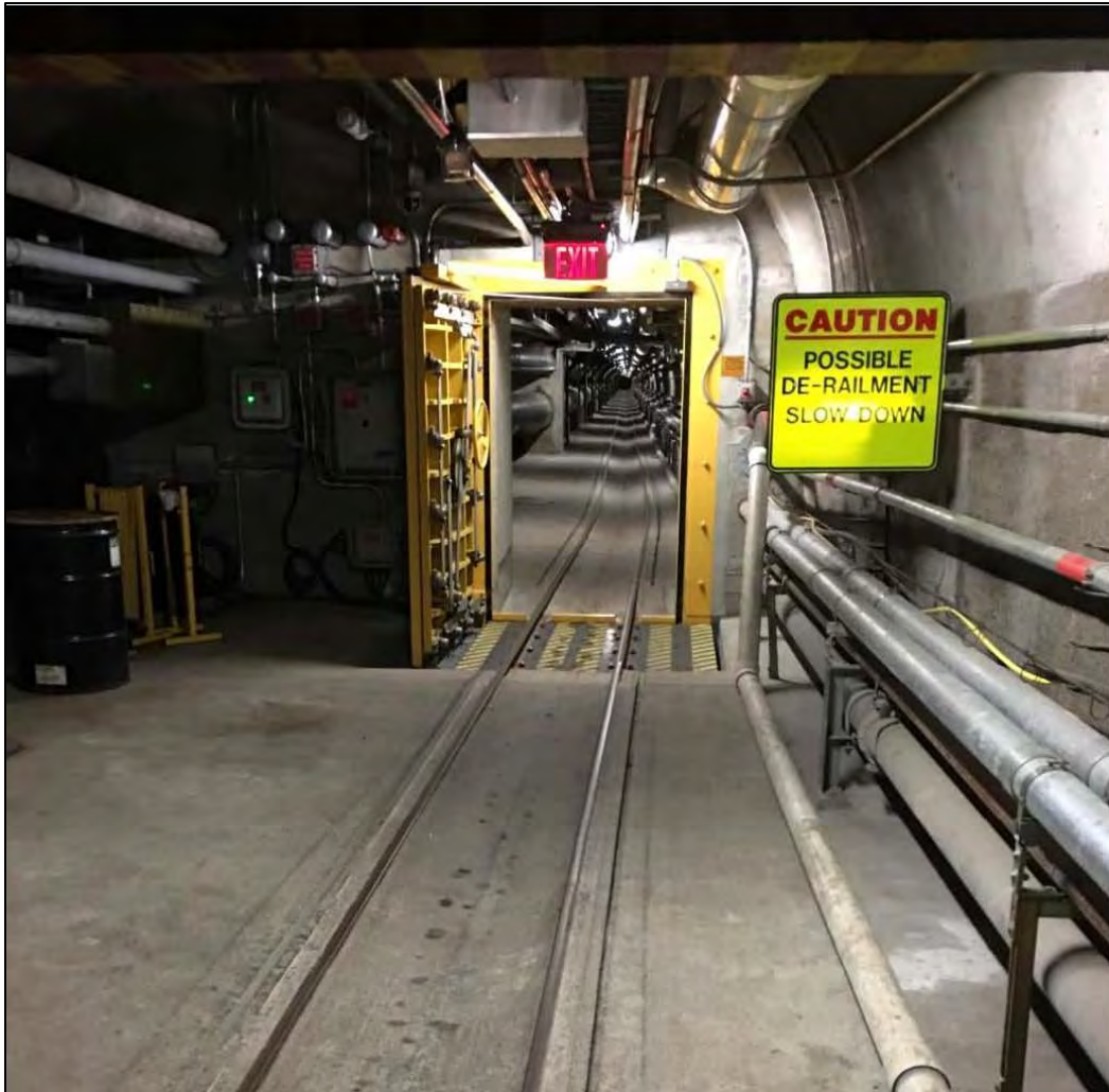
Figure 4.1: Emergency Oil Pressure Door
