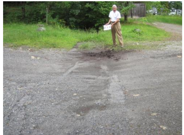
Improvements are needed at a commercial parking lot in Sector 20 to prevent sediment from getting into the lake.
