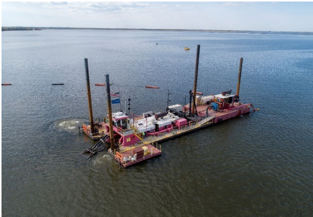
Historic PCB cleanup was completed in the Lower Fox River in 2020, marking a major milestone in AOC remediation work. Photo Credit: J.F. Brennan Company
