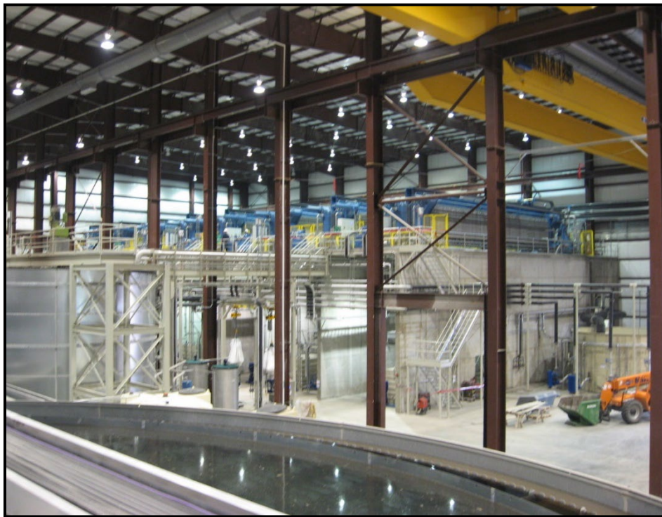
Figure 12. Clarifying tanks and presses in the treatment facility. Photo credit The Boldt Co.
