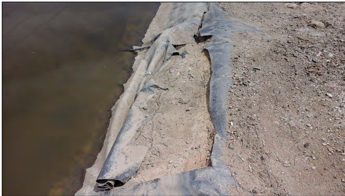
Photograph 21. Close-up view of the torn poly liner of Webber's Pond shown in Photograph 20.
