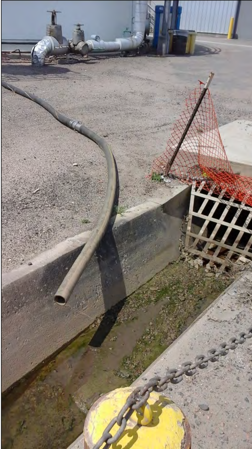
Photograph 17. Additional view of a decant line from the Tank B clarifier skimming collection tank shown in Photograph 16.
