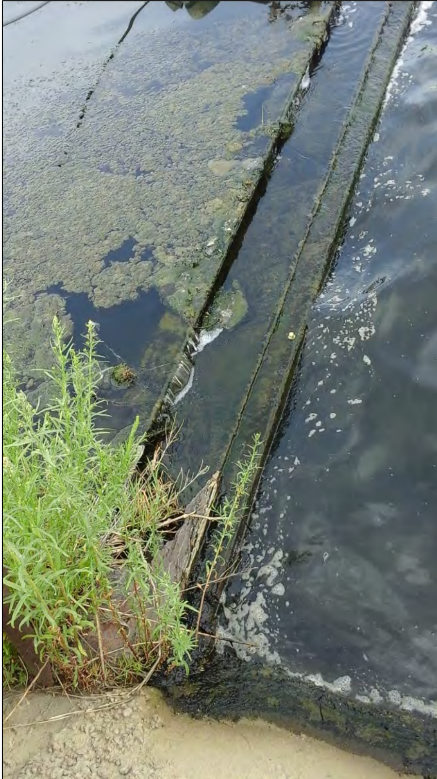
Photograph 11. View of accumulated solids and vegetative growth at the weir between Lagoon Nos. 1 and 2.
