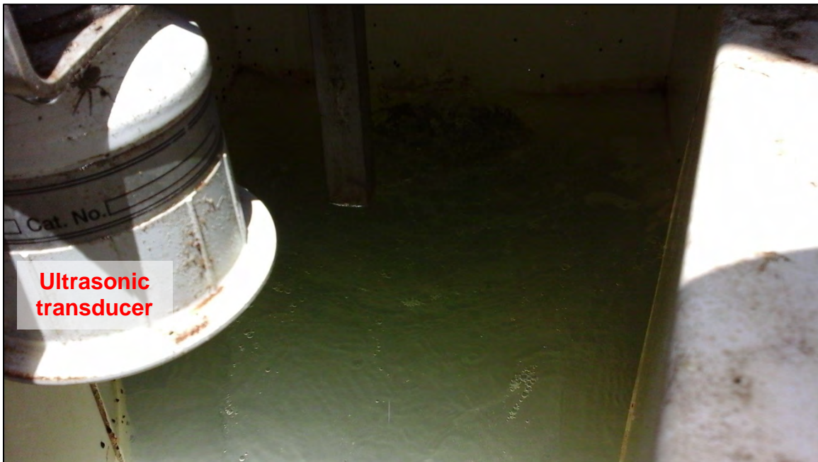
Photograph 14. View of the Outfall 003B Parshall flume and associated ultrasonic transducer for Permit flow measurements from the GWTS. Note the turbulence and disturbance (boils) observed in the approach channel run leading to the flume.
