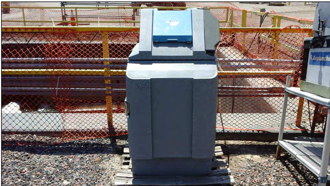
Photograph 4. View of the ISCO 4700 automatic sampler located at the Outfall 020A aerated sampling vault. This sampler was not equipped with an independently calibrated thermometer.
