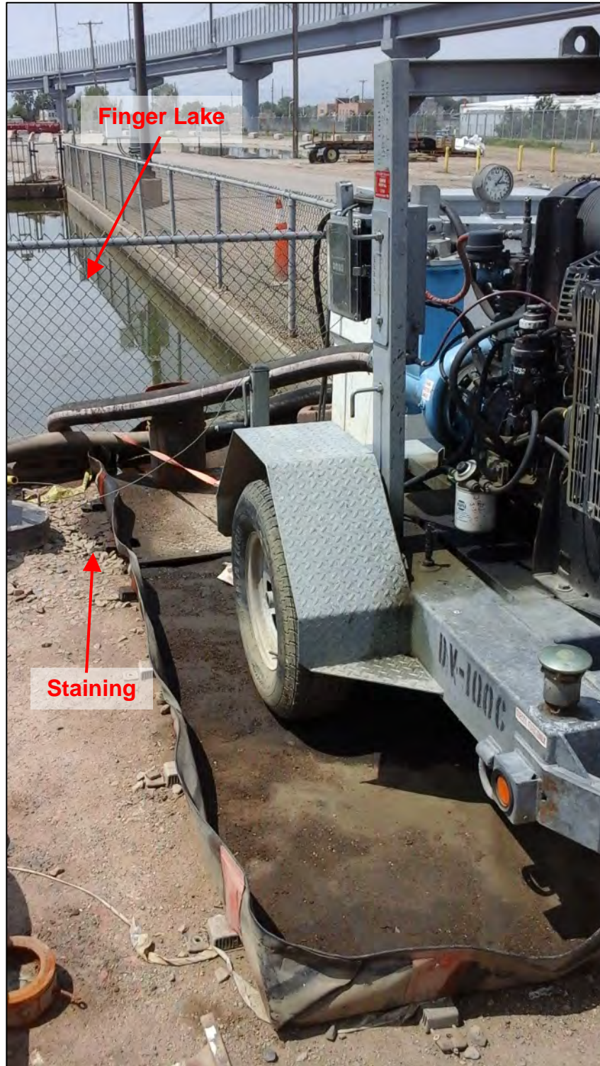
Photograph 22. View of the pump that transfers the contents of Finger Lake into Webber's Pond or to the WWTP. The pump was located within secondary containment; however, petroleum staining was observed on the ground surface outside of the containment.
