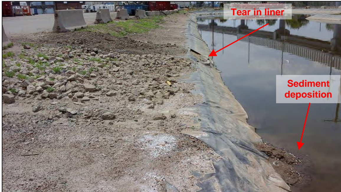
Photograph 20. View, facing south, of rill formations along the eastern embankment of Webber's Pond. Note the sediment deposited in Webber's Pond beneath the rill. Also note the torn poly liner for Webber's Pond, as shown in Photograph 21.
