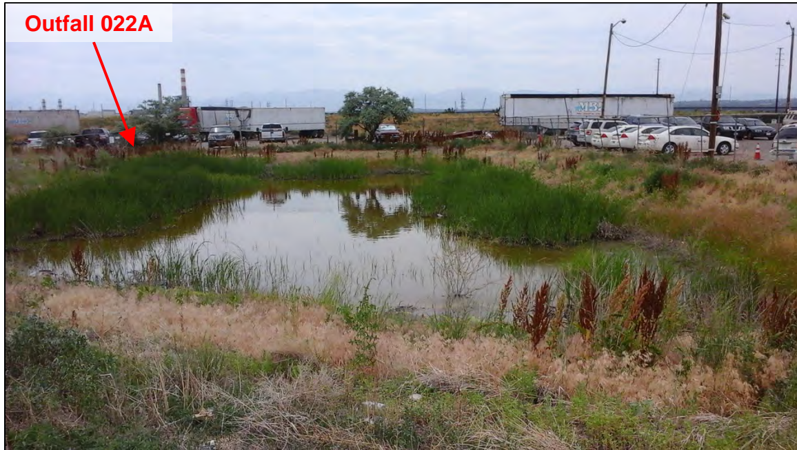
Photograph 16. View, facing west, of the stormwater detention basin located in the northwest corner of the Nelson Property. This basin discharges through Outfall 022A shown in Photograph 5. Note the significant vegetative growth potentially diminishing the capacity and effectiveness of this stormwater control.
