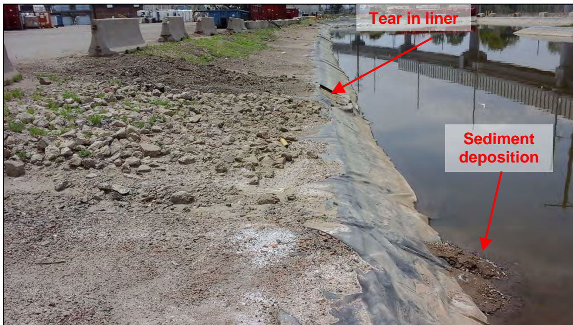
Photograph 33. View, facing south, of additional rill formations along the eastern embankment of Webber's Pond. Note the sediment deposited in Webber's Pond beneath the rill. Also note the torn poly liner for Webber's Pond, as shown in Photograph 36.
