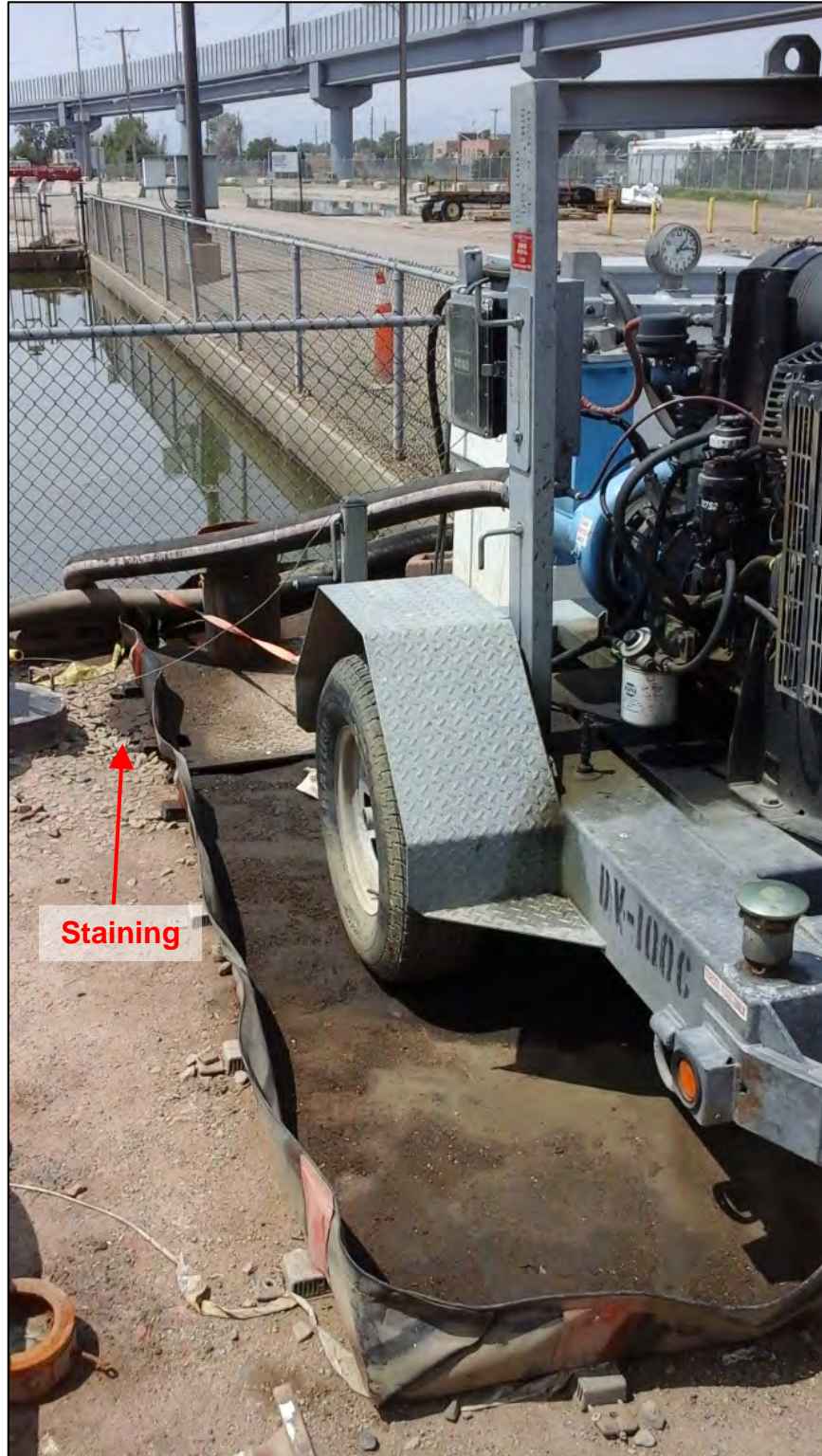
Photograph 20. View of the pump that transfers the contents of Finger Lake into Webber’s Pond or to the WWTP. The pump was located within secondary containment; however, petroleum product staining was observed on the ground surface outside of the containment.
