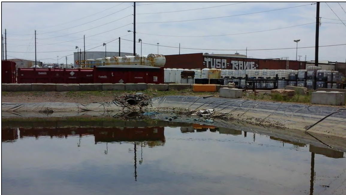
Photograph 19. View, facing southeast, of an inlet into the southeast corner of Webber's Pond. Not the trash and debris in the pond adjacent to this inlet.
