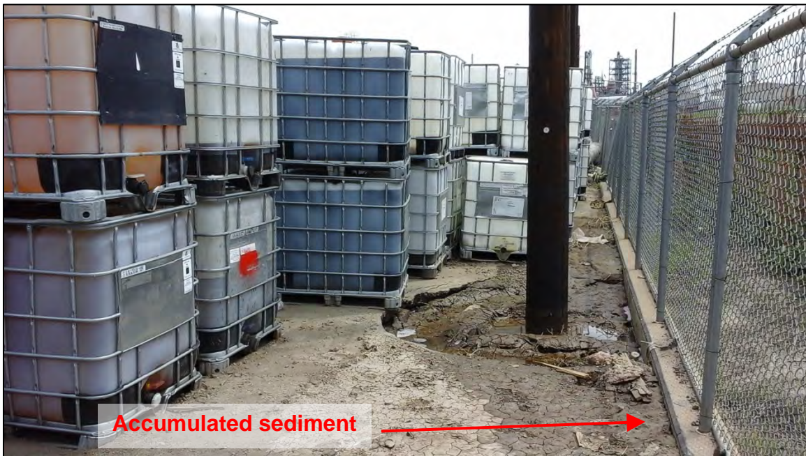
Photograph 26. View, facing north, of sediment accumulation against the Facility's south perimeter wall at the waste chemical and used oil storage area shown in Photograph 25. Note secondary containment was not provided for these totes of waste fluids.
