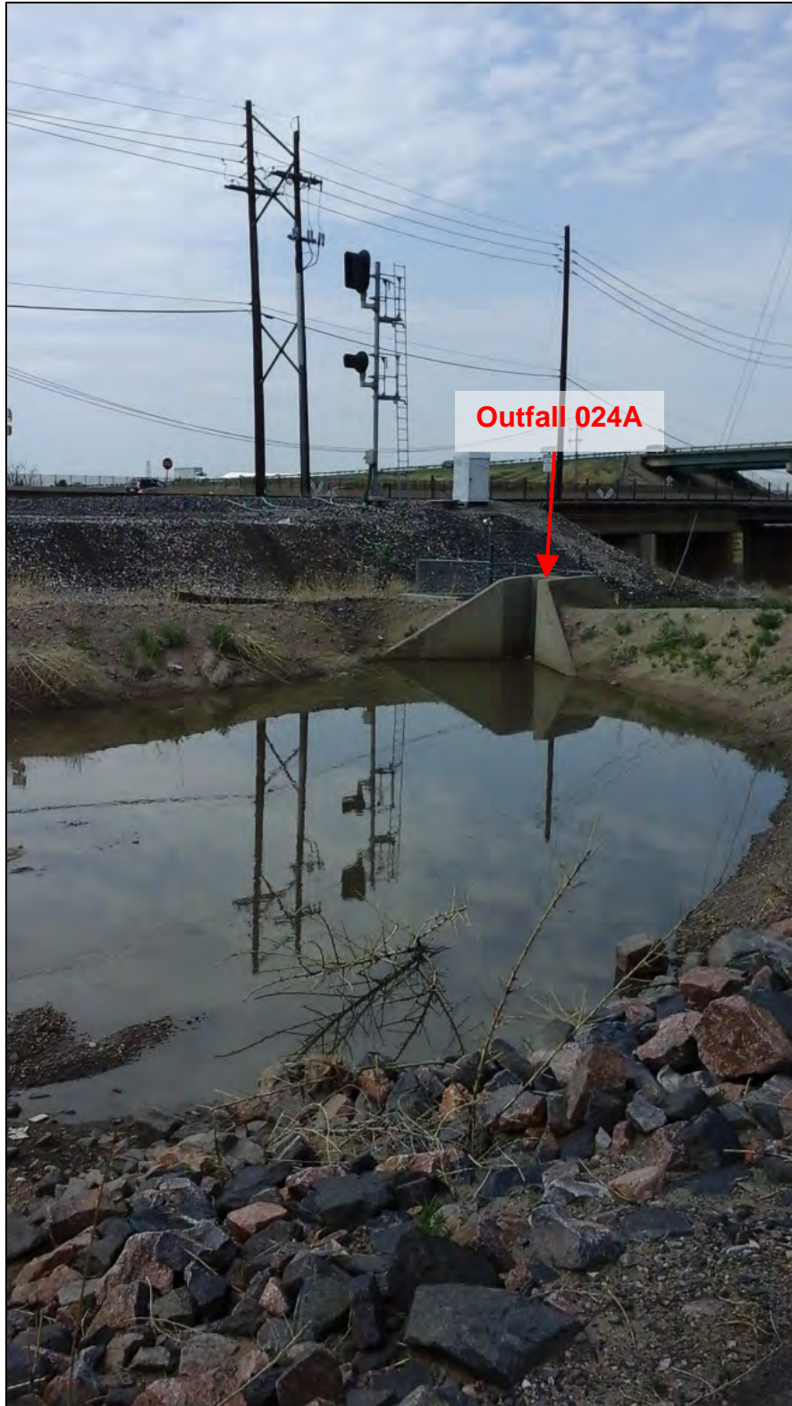
Photograph 9. View, facing northwest, of Outfall 024A downgradient of a stormwater detention basin that captures runoff from the Plant 2 employee parking lot.
