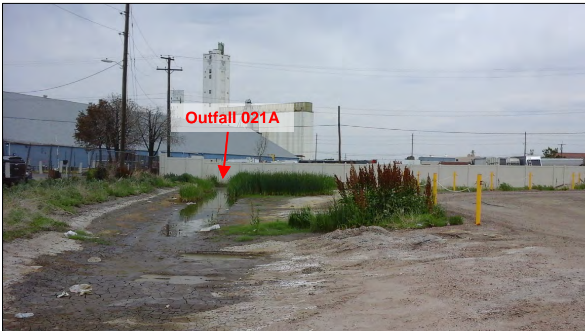
Photograph 14. View, facing east, of the stormwater detention basin in the northeast corner of the Nelson Property which discharges to Outfall 021A (refer to Photograph 3). Accumulated sediment and vegetative growth was observed within the basin.
