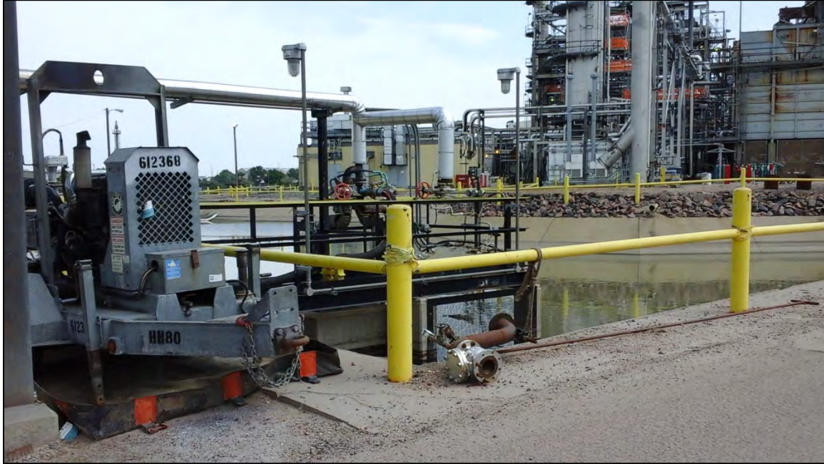
Photograph 23. View of the pump that transfers the contents of Mary's Pond to the WWTP during normal conditions.
