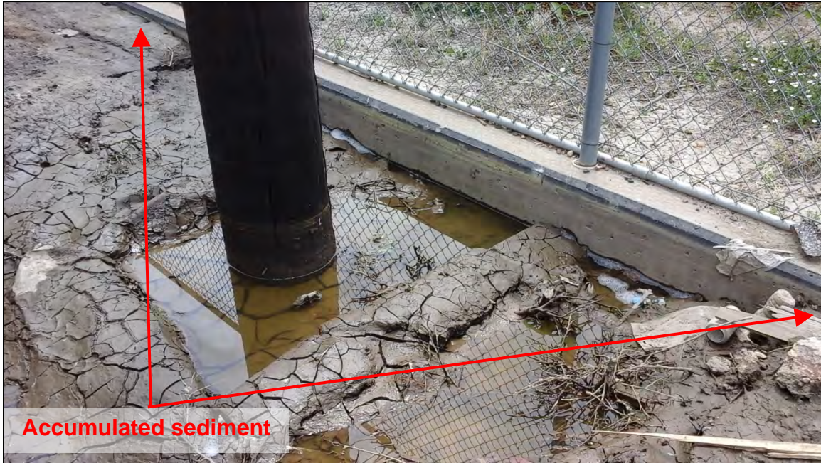
Photograph 27. Additional view of accumulated sediment along the south perimeter wall shown in Photograph 26. Note the depth of sediment varied along this perimeter wall.
