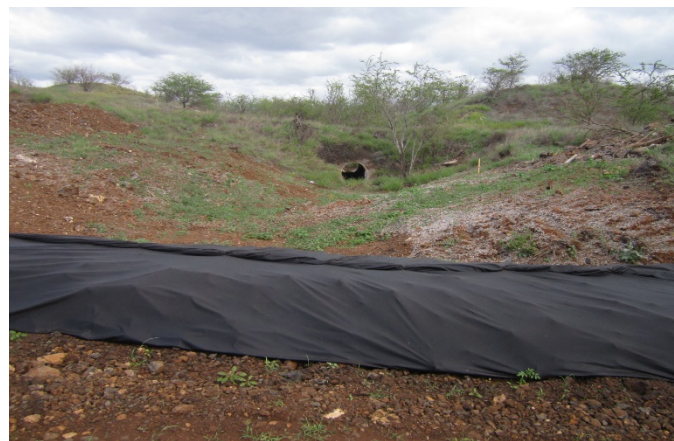
A gravel filter berm covered with filter fabric.
