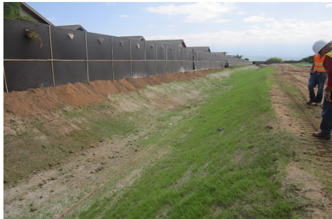
Grass-lined channel in a construction area.
