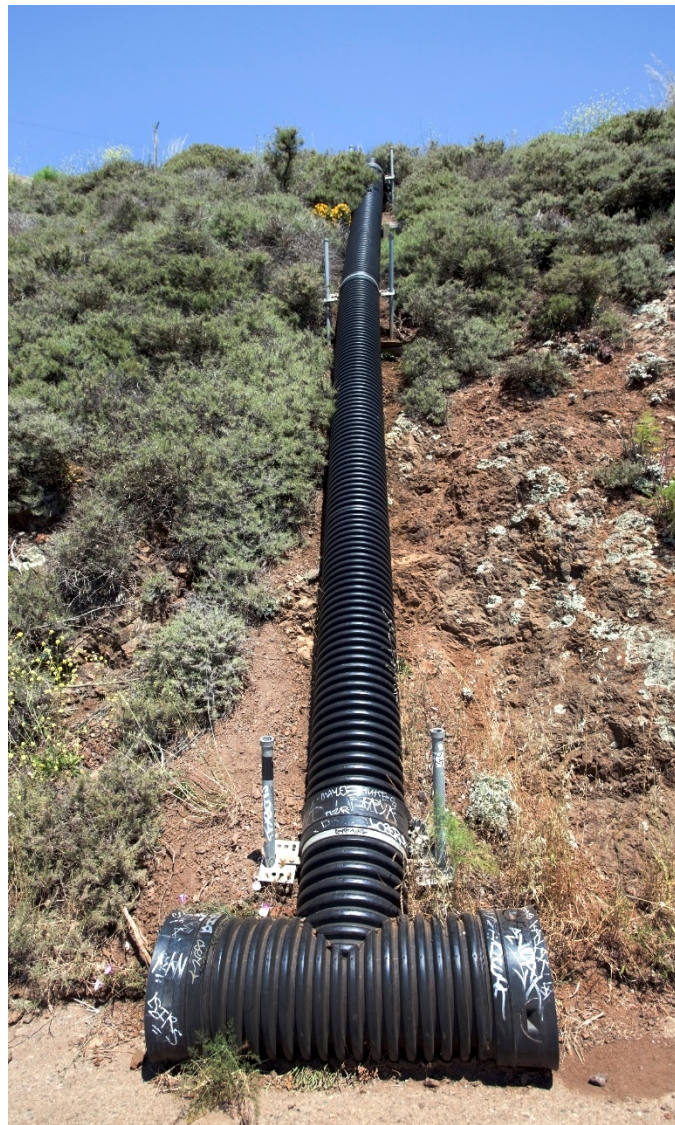
A temporary slope drain made from corrugated pipe. A “T” fitting at the downstream end slows discharge and prevents erosion.
