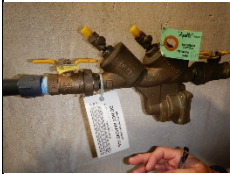
12: DSCN0353JPG Location: Benton Harbor PWS Photographer: Naomi Huff Date/Time: 9/21/2021 9:38 AM
