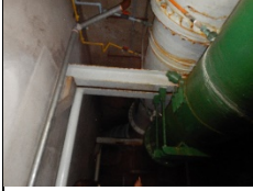
10: DSCN0343JPG Location: Benton Harbor PWS Photographer: Naomi Huff Date/Time: 9/21/2021 9:34 AM
