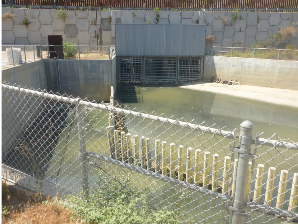
Figure 4-5. Photograph of the Goat Canyon flow diversion structure, taken by PG Environmental on May 27, 2021.
