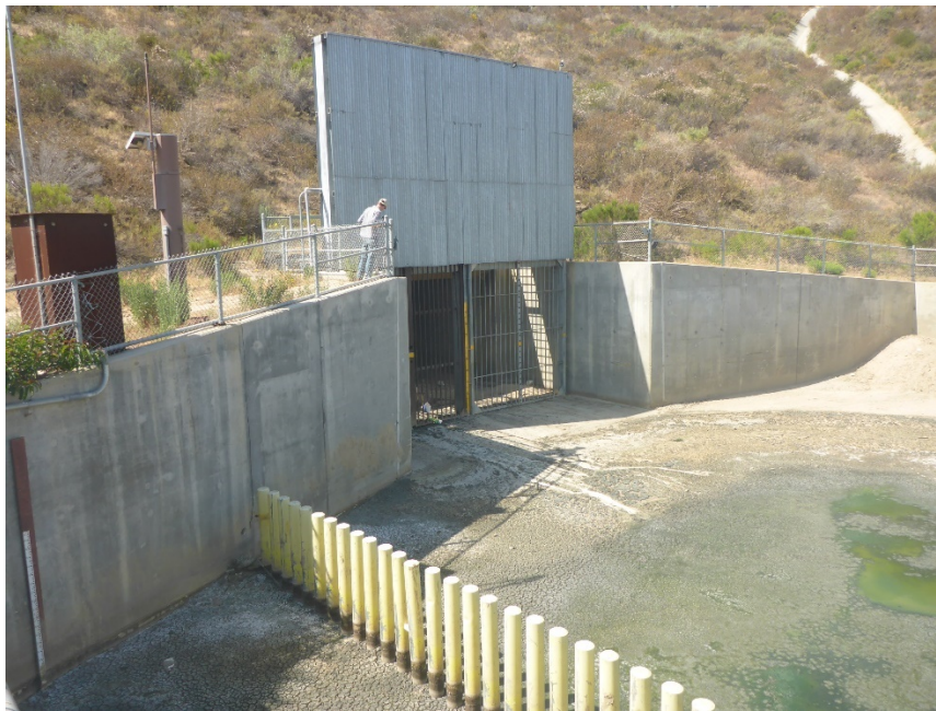
Figure 4-4. Photograph of the Smuggler's Gulch canyon flow diversion structure, taken by PG Environmental on May 27, 2021.
