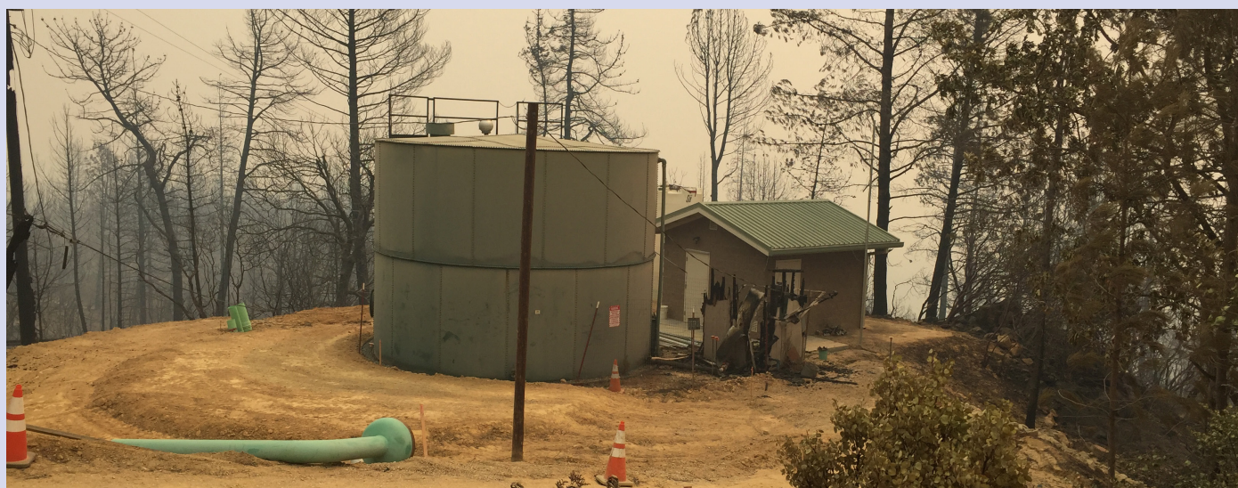
Source: PACE Engineering, Shasta CSD Upper Brunswick Pump Station alongside remains of the old wood frame pump station after the fire.
