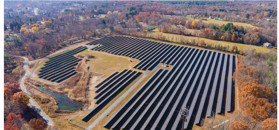
The 6140 Route 209 Solar Site, Kerhonkson, NY. Photo credit: Nexamp .
