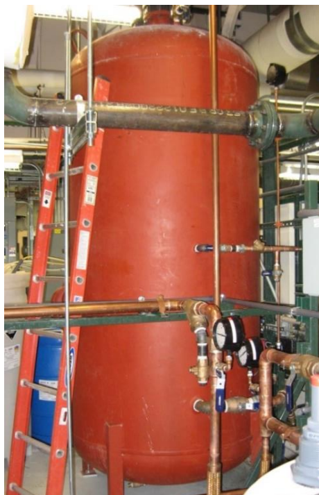
Photograph - NPDES-03A199-18-006 LDCC Neutralization Tank
