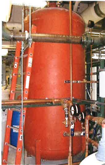
Photograph - NPDES-03A199-18-006 LDCC Neutralization Tank
