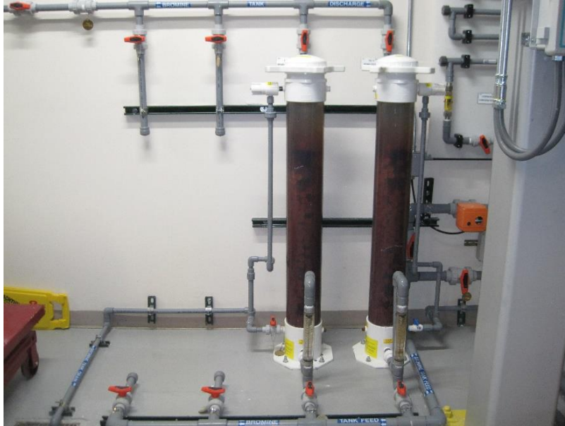
Photograph - NPDES-03A027-18-012 SCC Trinity Cooling Towers - Brominators
