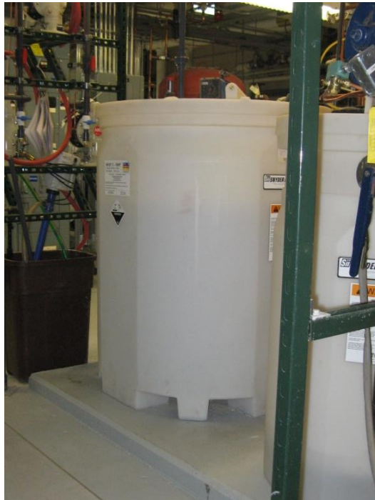
Photograph - NPDES-03A199-18-005 LDCC Corrosion Inhibitor and pH Adjustment Chemical Feed Tanks
