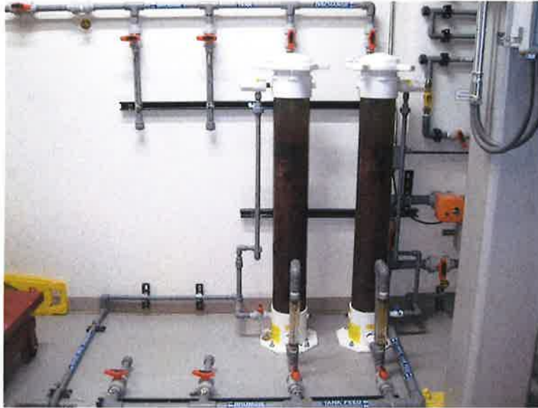
Photograph - NPDES-03A027-18-012 SCC Trinity Cooling Towers - Brominators
