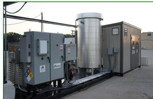
BioCNG System Dane County, WI
