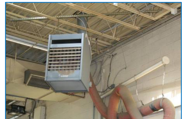
Infrared Heater - Lorton, VA
