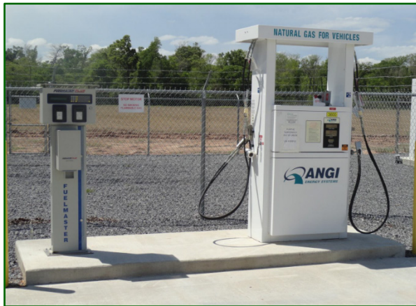
CNG Fueling Station St. Landry Parish, LA
