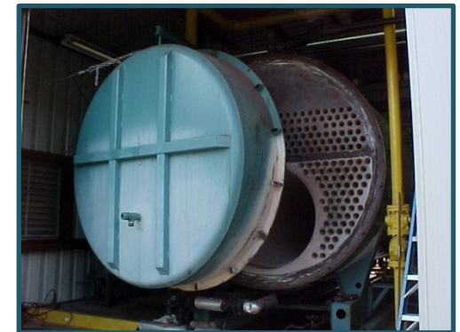
Boiler – Raleigh, NC
