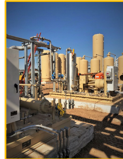
RNG Plant – Phoenix, AZ
