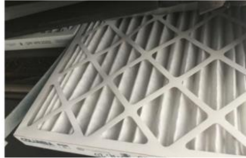
Clean HVAC filter
