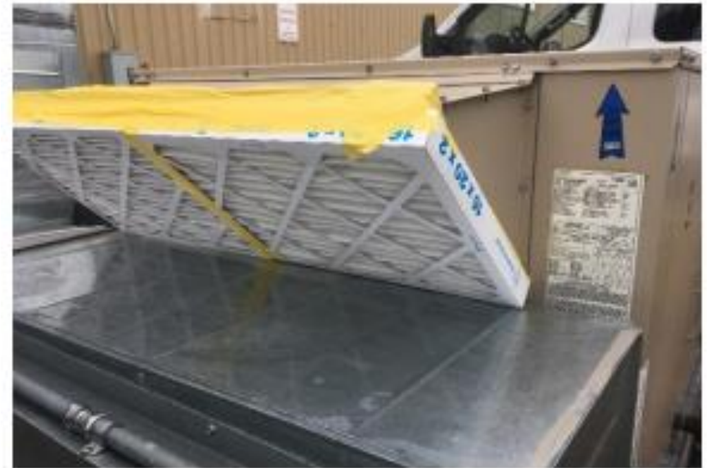
Supplemental filtration with a MERV13 filter installed on an outdoor air intake
