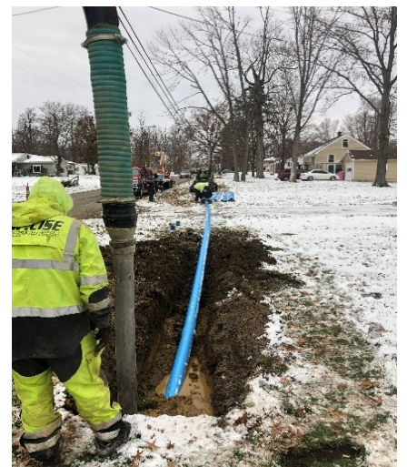
A worker oversees slurry being vacuumed from the boring pit while others assemble sections of pipe to lay.
