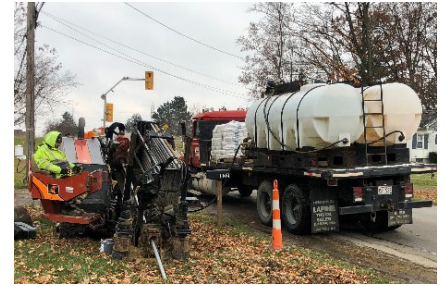
An operator uses a horizontal directional drill to bore the initial pilot hole and begin clearing a path for the water main.
