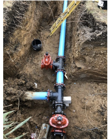
Workers assemble fittings, gate valves, and restraining joints along the water main.
