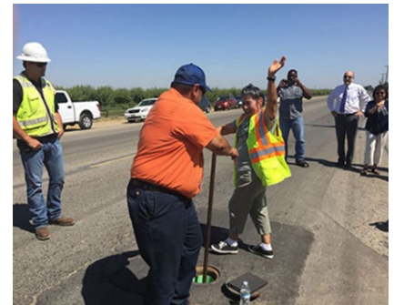
A Matheny Tract resident opens the water valve to bring safe reliable drinking water to the community.
