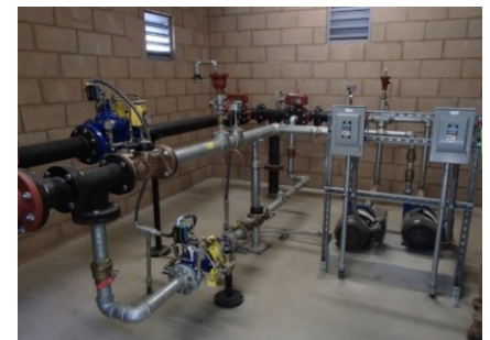
Booster pumping station.
