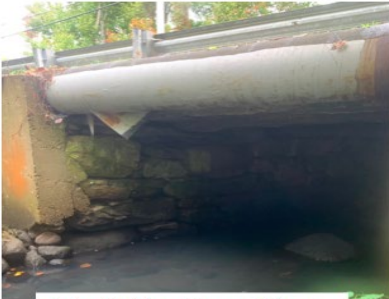
Aging Highland Street Culvert
