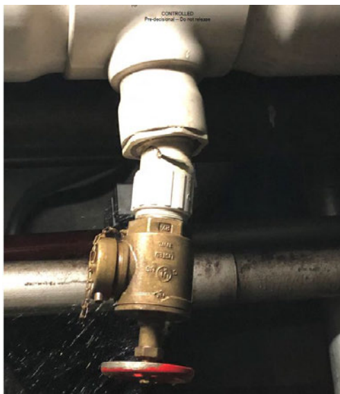
Cracked Low Point Drain
