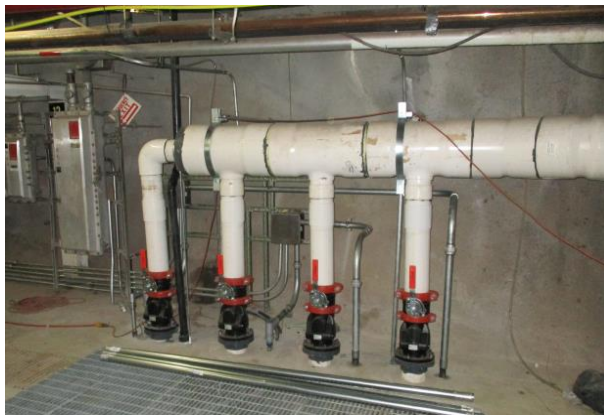
Original AFFF Retention Line Piping in Immediate Area of an AFFF Sump
