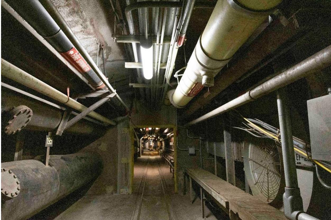
Lower Access Tunnel with AFFF retention line in top right (PVC pipe)
