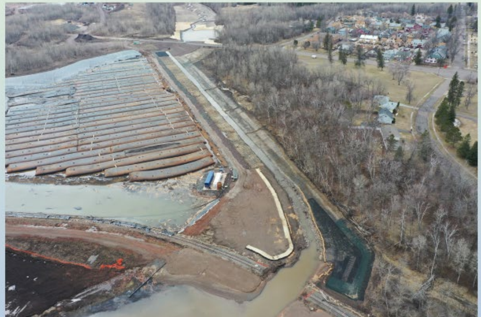
In progress: Photograph of the Upland CDF facing Spirit Lake during remediation.
