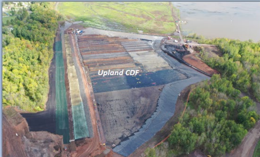
In progress: Photograph of the Upland CDF facing Spirit Lake during remediation.
