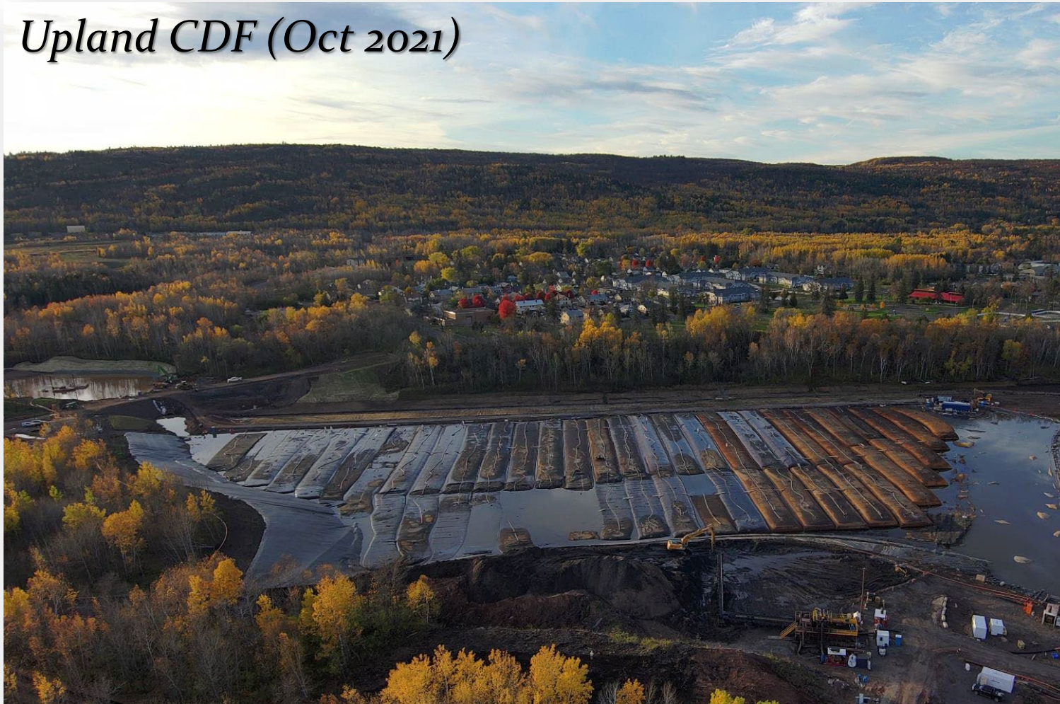
Week of Oct. 25, 2021, Photo #2: An aerial view of the Upland confined disposal facility (CDF) and Geotubes®. (10/11/2021))
