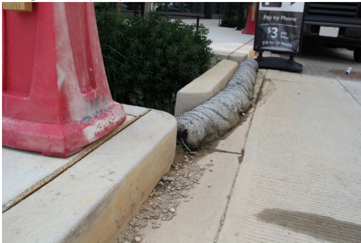
Figure 19-4. View of filter sock covering inlet to bioretention cell along First Street.
