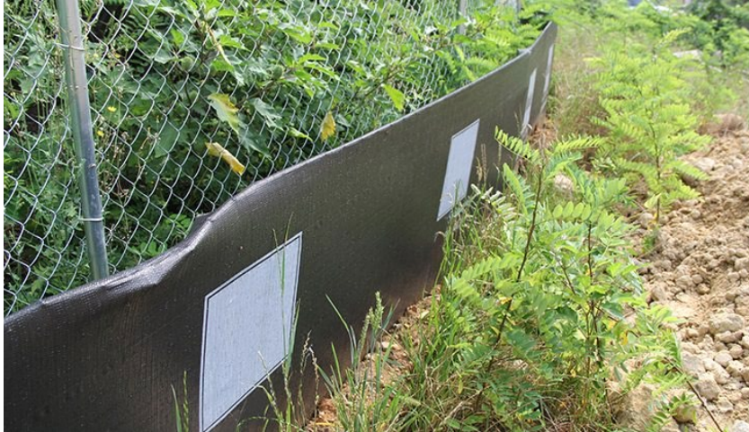
Figure 12-5. View of a different section of the silt fence upgradient of the stockpile.
