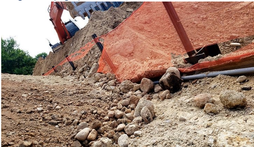
Figure 14-6. View of orange safety fence immediately downgradient of the soil stockpile, above the active construction area.
