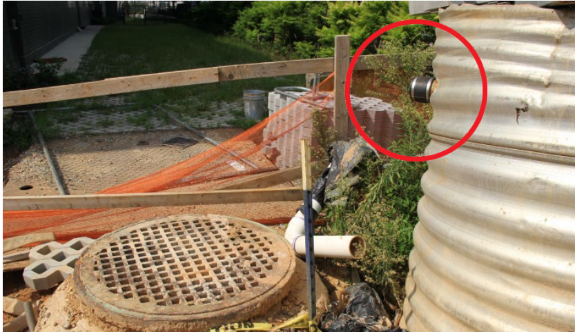
Figure 16-6. View of the outlet of the portable sediment tank.
