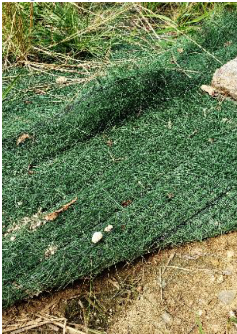
Figure 15-4. Displaced erosion control matting on the diversion berm.
