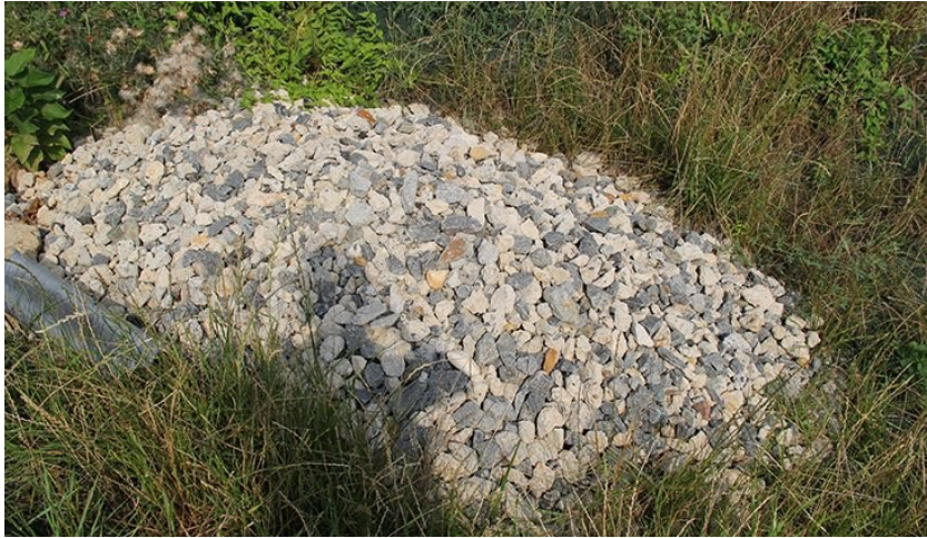
Figure 15-7. View of check dam at the downgradient end of the area contained by the diversion berm.
