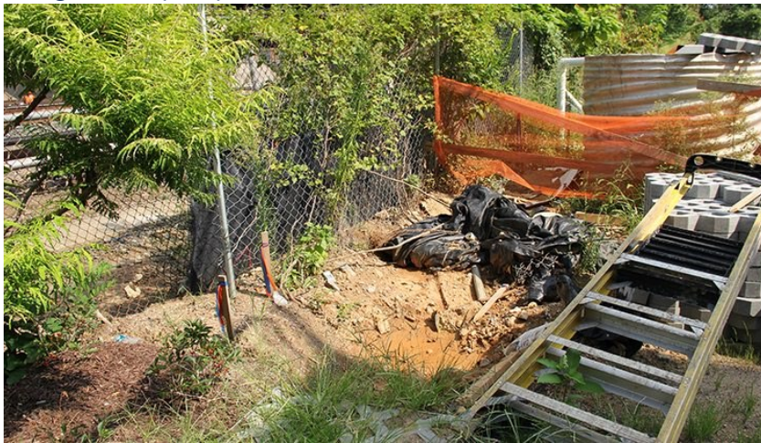
Figure 17-3. Debris and construction materials on the ground near the portable sediment tank.
