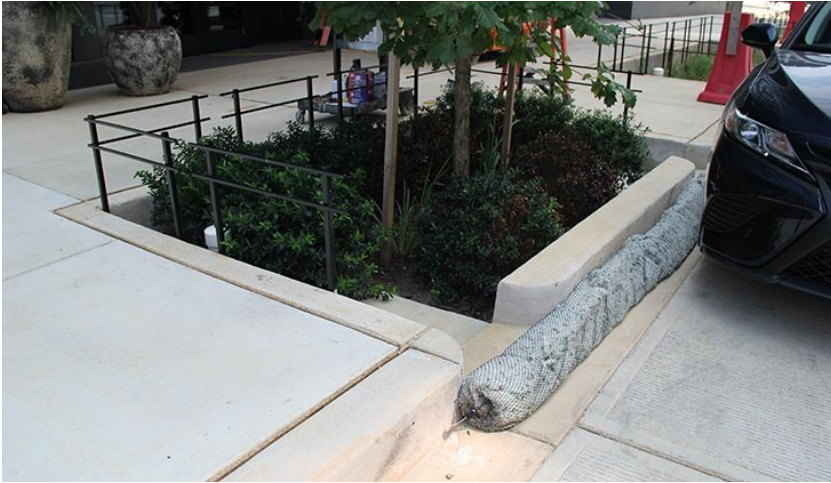
Figure 20-4. View of second bioretention cell along First Street.
