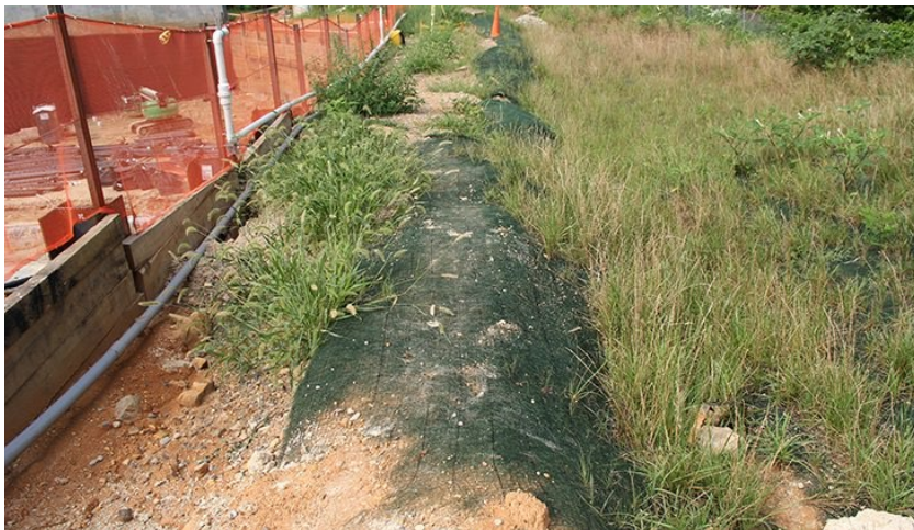
Figure 14-4. View of the diversion berm along the perimeter of the active construction area.
