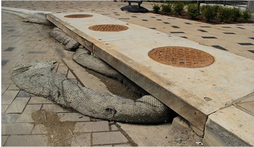
Figure 22-5. View of the filter sock in the curb inlet at the end of First Street.
