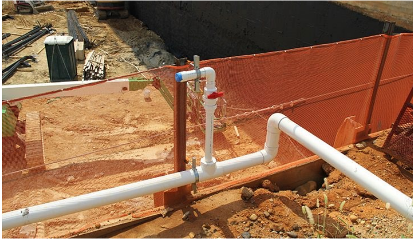
Figure 16-4. Piping and a valve that are part of the dewatering system for the active construction area.
