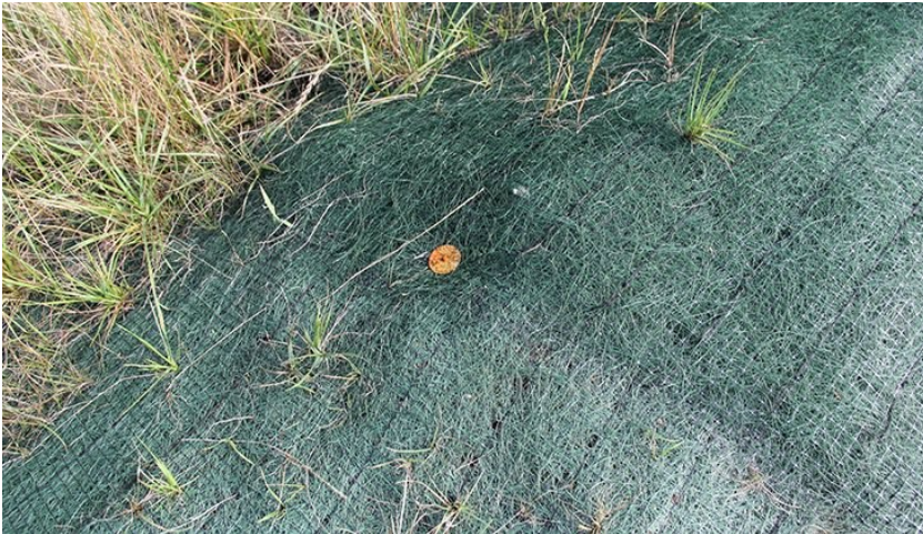
Figure 15-6. The erosion control matting is anchored to the diversion berm with nails.
