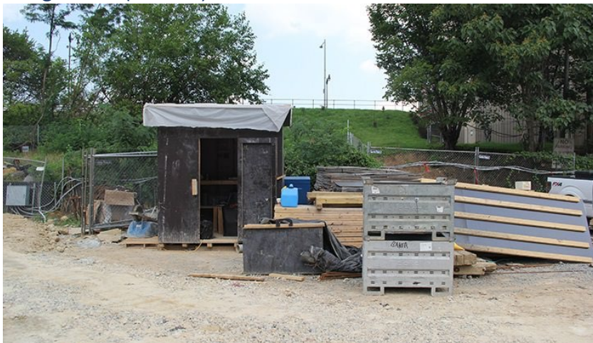
Figure 11-5. View of materials storage area near the entrance to the active construction area.
