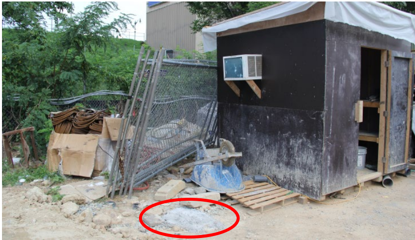
Figure 11-4. Improper concrete washout next to a storage shed.
