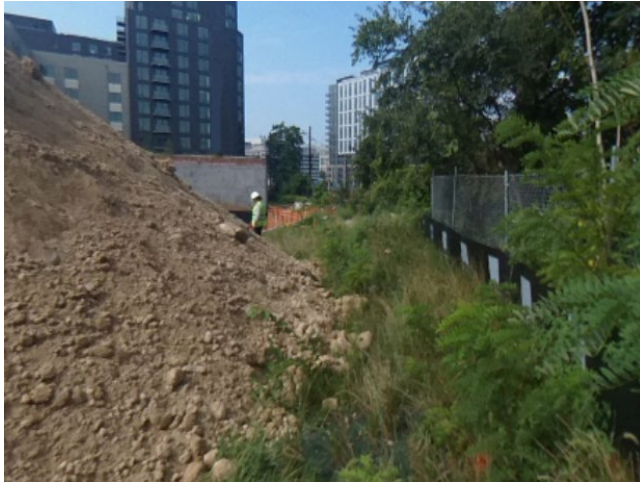
Figure 13-4. View of the soil stockpile and a section of silt fence upgradient of it.
