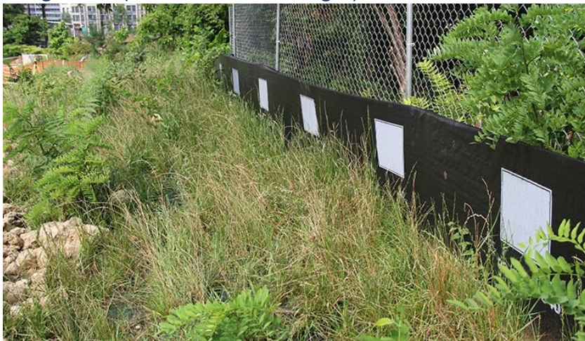
Figure 12-4. View of a section of silt fence along the site perimeter upgradient of the stockpile.
