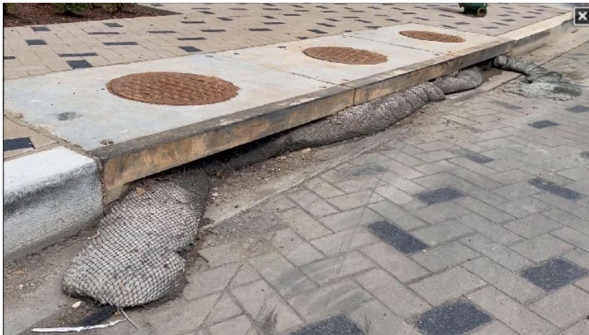
Figure 22-4. Screenshot of a video showing the condition of the filter sock in the corner curb inlet.
