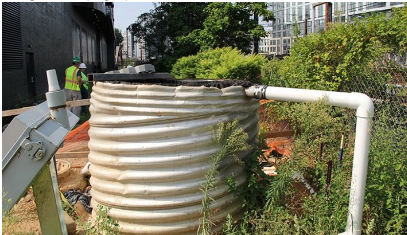
Figure 16-7. View of the inlet pipe leading into the portable sediment tank.
