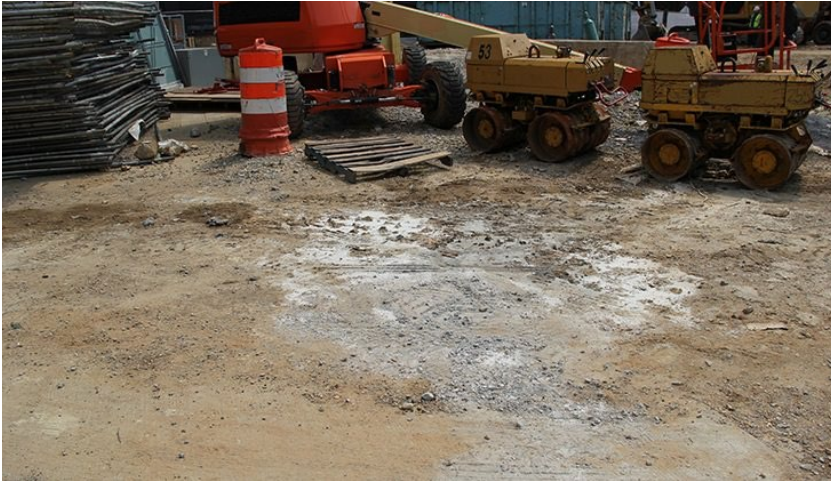
Figure 11-7. Concrete washout on the ground in the materials storage area.
