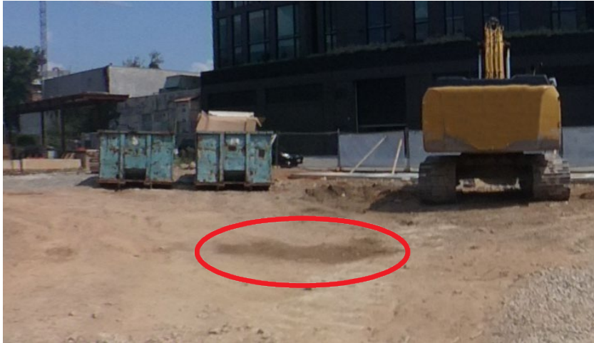
Figure 4-9. There is a grease stain on the ground in the materials storage area.
