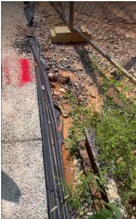
Figure 16-4. Screenshot of video showing collapsed silt fence along Second Street.
