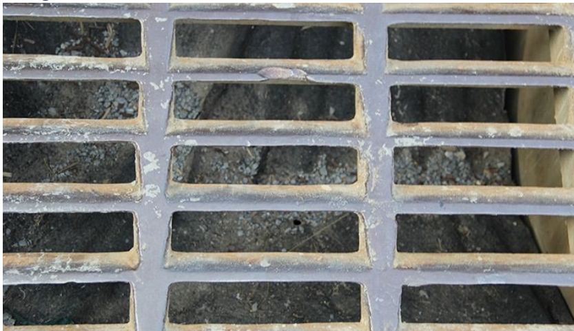
Figure 17-4. Close-up view of storm drain at the intersection of Second Street and Main Street.
