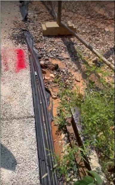
11. A collapsed silt fence along Second Street.
