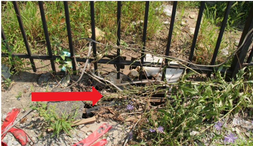
Figure 14-4. View of storm drain at the end of the materials storage area.
