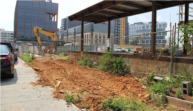
10. A freshly disturbed area with no perimeter controls along Second Street.
