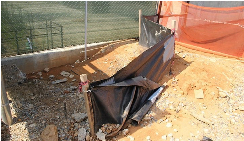
Figure 2-5. Another view of the silt fence in the area behind the truck.
