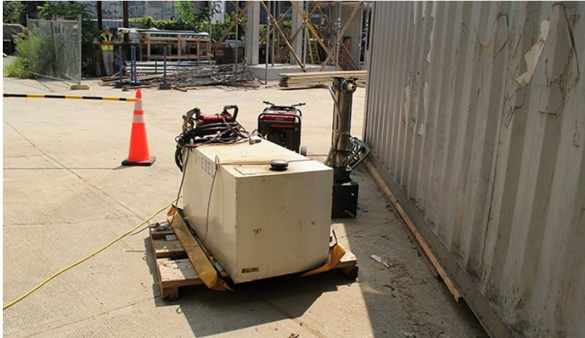
Figure 13-5. View of the back of the large fuel tank.
