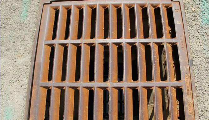
12. An unprotected storm drain inlet on Second Street.
