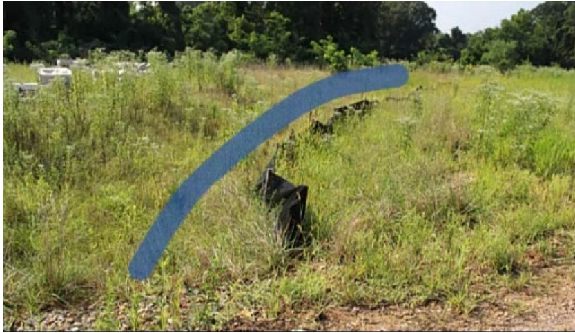
Figure 12-5. Silt fence along the upgradient side of the grass swale.
