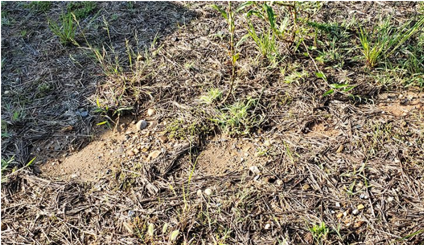
Figure 10-4. Close-up view of bare area on the large stockpile.
