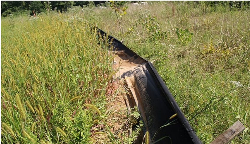
Figure 13-4. View of collapsed silt fence along the grass swale.
