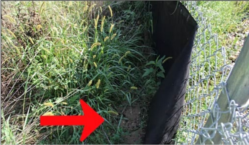
Figure 7-5. View of super silt fence downgradient of the sediment trap outlet.
