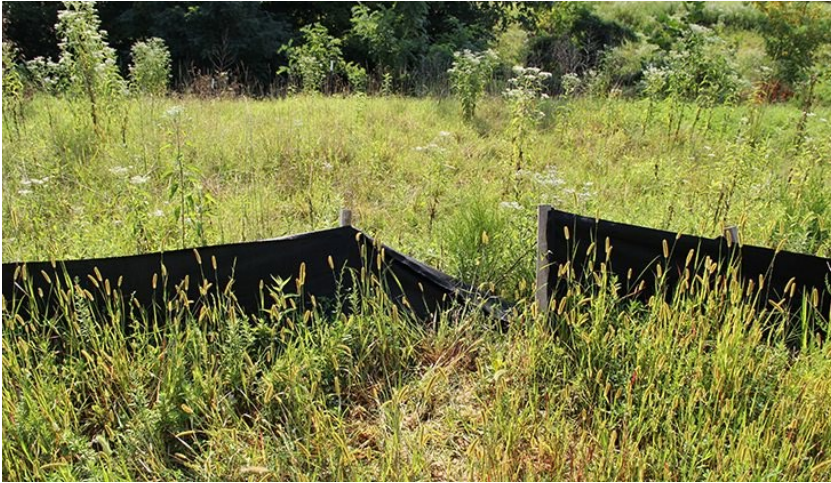
Figure 13-5. View of detached filter fabric on the silt fence along the grass swale.
