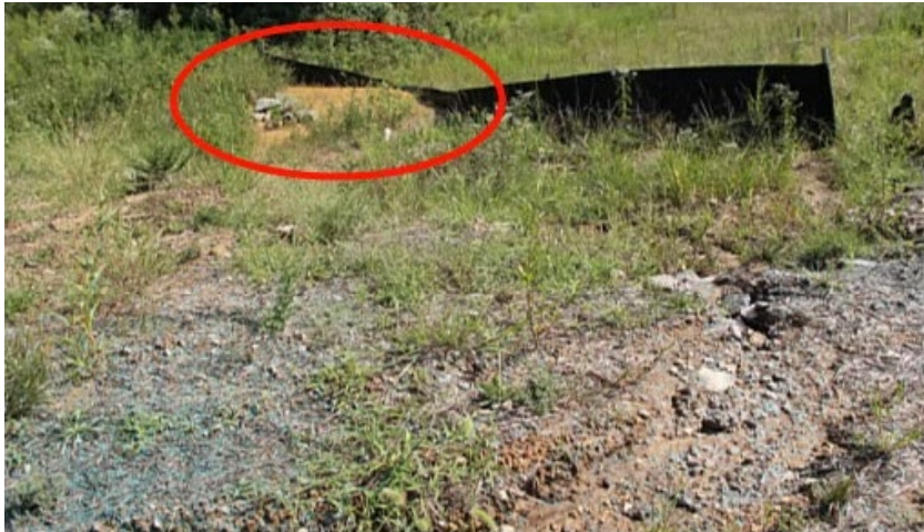
Figure 9-6. View of eroded stockpile slope upgradient of silt fence.
