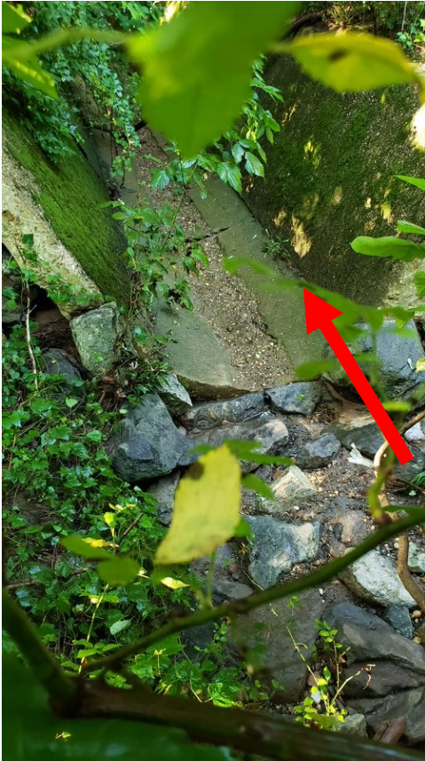
Figure 14-5. View of the downstream side of the sediment trap's outlet, and the concrete channel downgradient of the outlet.
