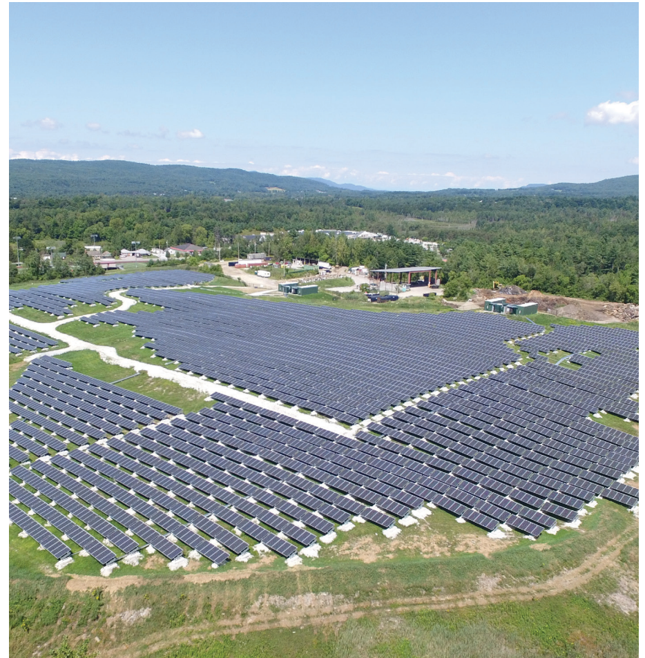
The Stafford Hill Solar Farm in Rutland, Vermont is a great example of solar on landfill with a 2.3 MW solar PV installation on 9 acres.
