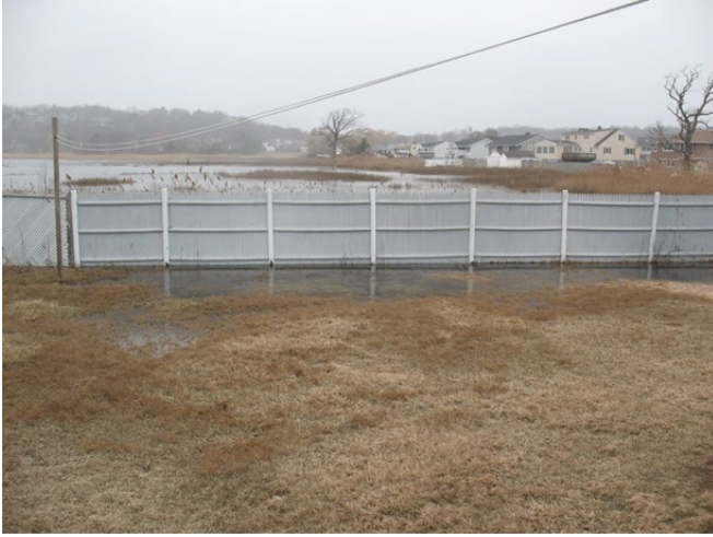
Figure C-21. March 30, 2018, high tide estimated at elevation 6.2 feet NAVD88. Photo credit Fae Saulenas.
