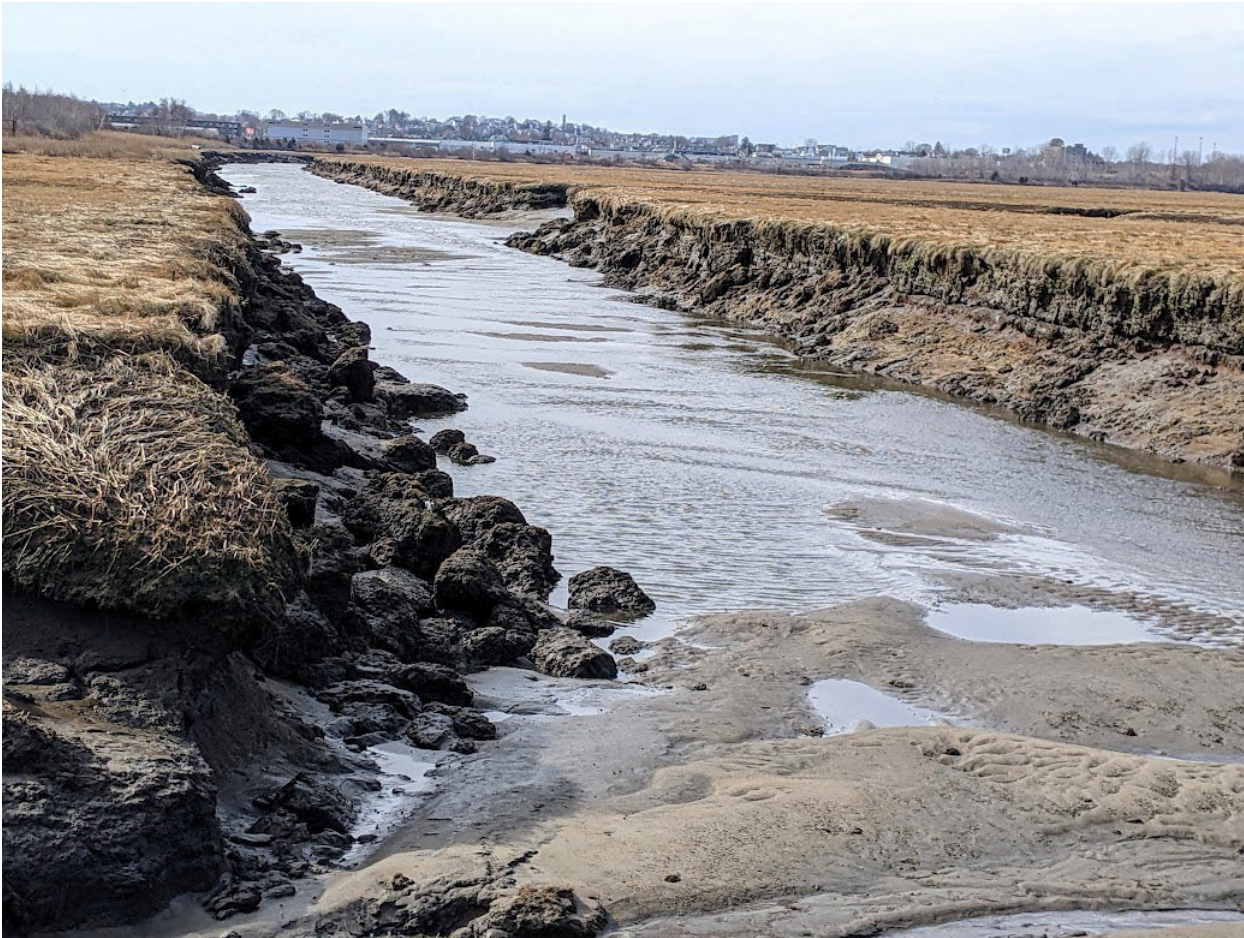
Figure 13. Photograph of the constructed “temporary” drainage channel in East Saugus looking south toward Revere taken February 23, 2022. The channel in some places is more than twice the original constructed width due to erosion of the salt marsh peat banks. Photo credit Ed Reiner.
