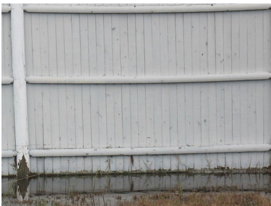
Figure C-8. April 30, 2021. Debris on fence 16 inches high estimated at elevation 6.9 feet NAVD88. Photo credit Fae Saulenas.
