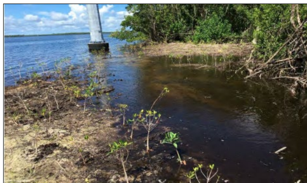
Figure 5- Example of a shallow water impact- installation of poles for power lines. Photo from a Jacksonville district permit.
