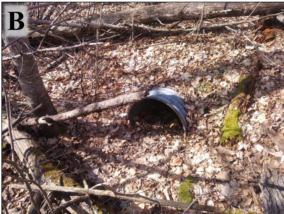
Plate 3. Example jurisdictional break evaluation depicting A) a roadway culvert that exhibits characteristics of at least seasonal surficial flow (ordinary high water marks (OHWM), vegetation preclusion, scour, etc.), and B) a roadway culvert that does not exhibit characteristics of at least seasonal surficial flow. Photos taken by LLBO staff in April 2020.
