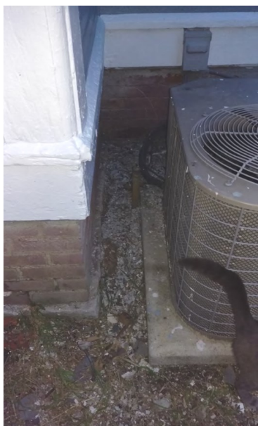
Lead-containing paint chips from improper removal cover the ground.
