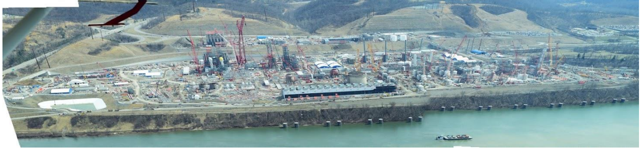
New Shell ethane cracker and polyethylene plant under construction on the Ohio River in Beaver County, Pennsylvania, with plans to be online in 2021. Photo credit: Ted Auch. 2019. Provided by FracTracker Alliance, fractracker.org . Aerial assistance provided by LightHawk, lighthawk.org .
