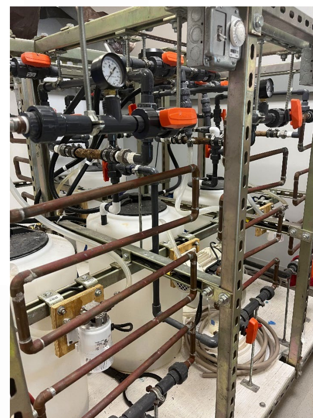
Figure 10 Pipe loop at NJIT using harvested lead-lined galvanized pipes.
