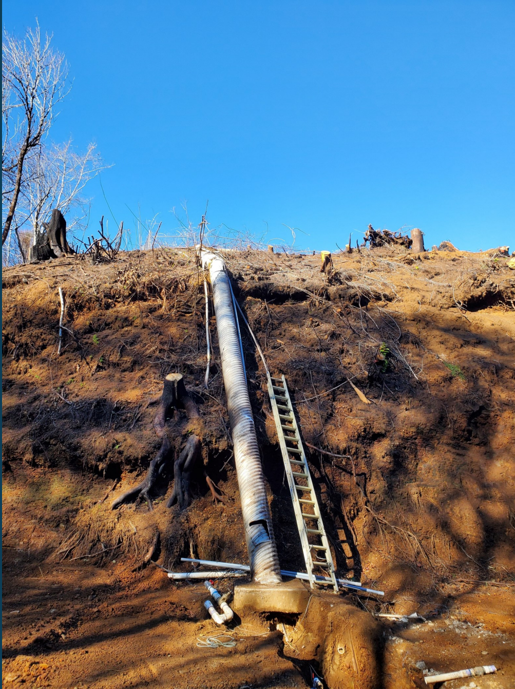
Wildfire damage to the embankment above water treatment plant
