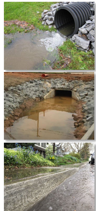
Examples of stormwater conveyance assets.
