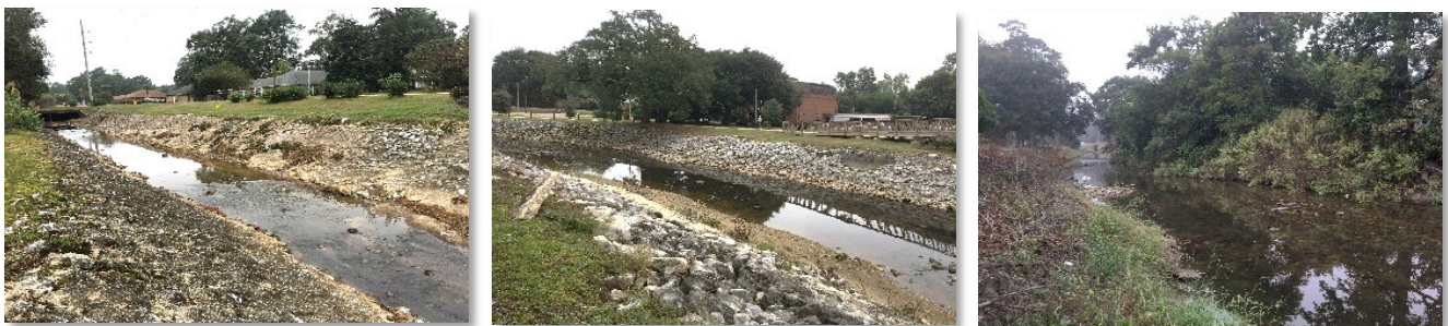
Left and middle images show rip rap and concrete armoring along Gordon's Creek. Right image shows a portion of Gordon's Creek without armoring.
