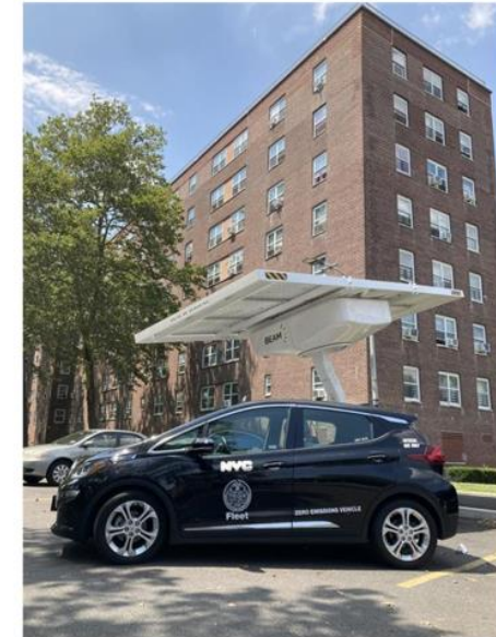
DCAS solar carport and shared Bolt at Sotomayor Houses in the Bronx.
