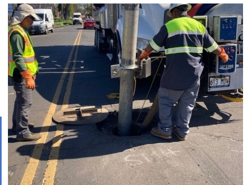
Figure 2. EPA contactors injecting water into a sewer pipe to remove any debris/blockages.
