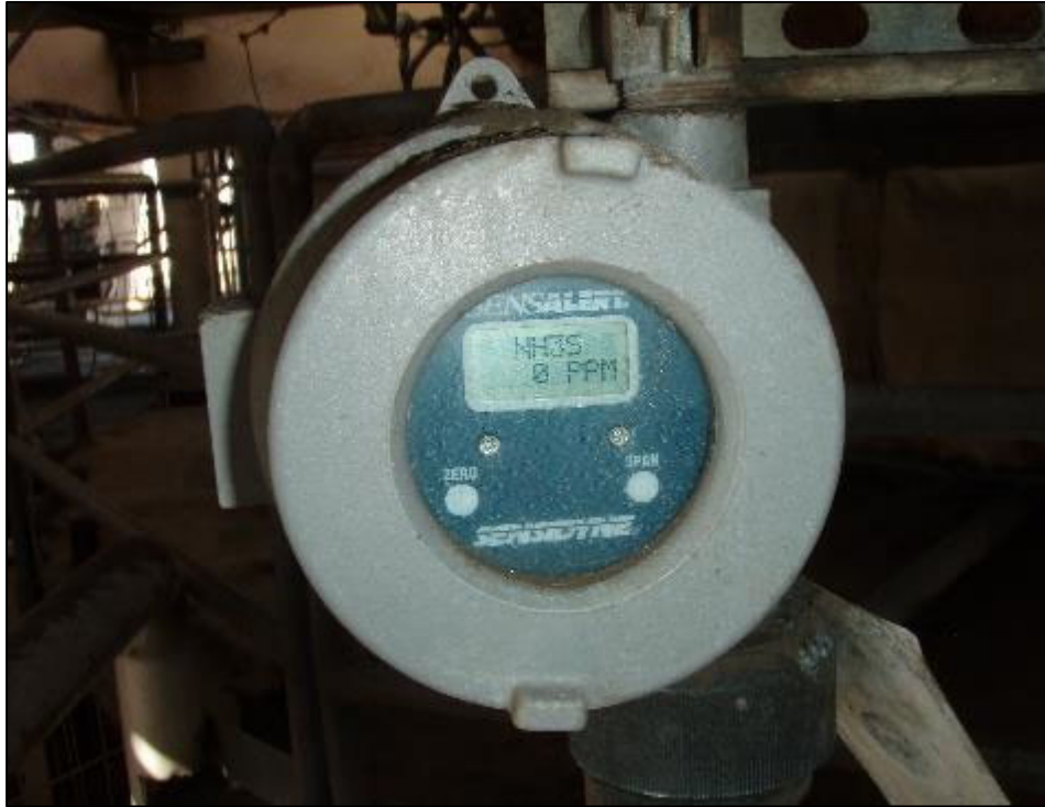
Photograph 3: View of Sensidyne gauge showing 0 ppm of ammonia at the SNCR unit.
