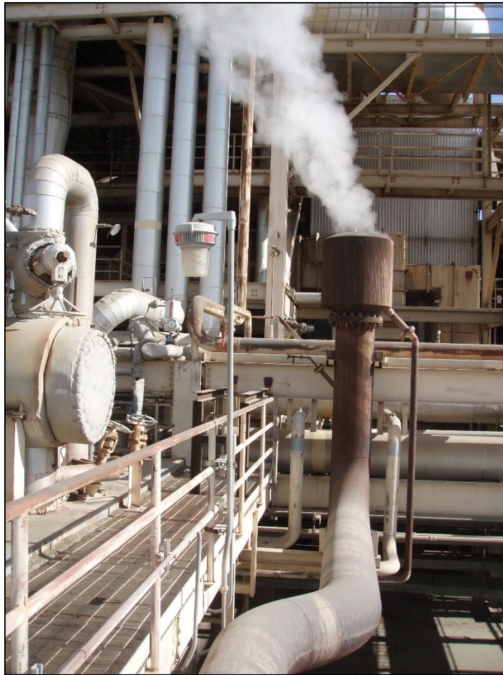
Photograph 9: View of blowdown vent and nearby equipment surfaces.
