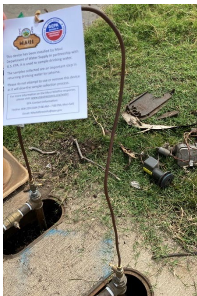
Figure 2. Meter box with apparatus and informational tag.
